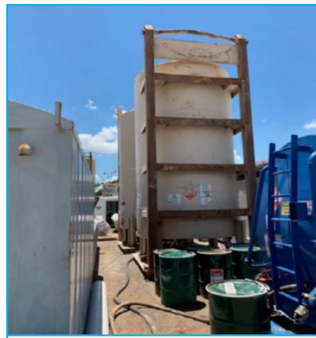
Upright Storage Tanks
