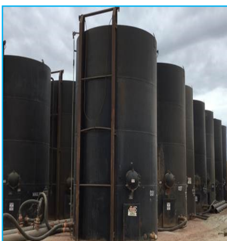
Upright Storage Tanks
